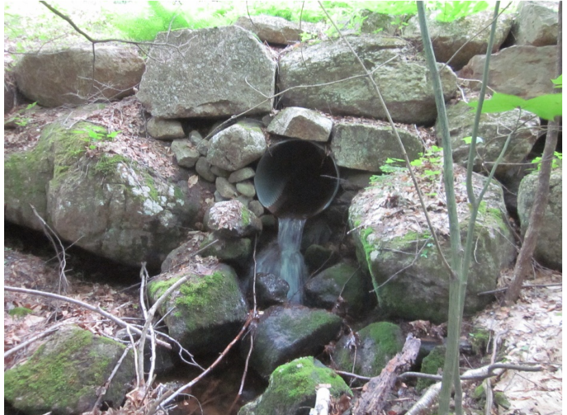
A culvert along the higher reaches of a tributary to Andrew Brook in Newbury. We visited several of these types of stream crossing structures to determine if fish are still present in the upper extent of these watersheds. At this location, twenty wild brook trout were captured below the culvert and no fish were found on the upstream side.
